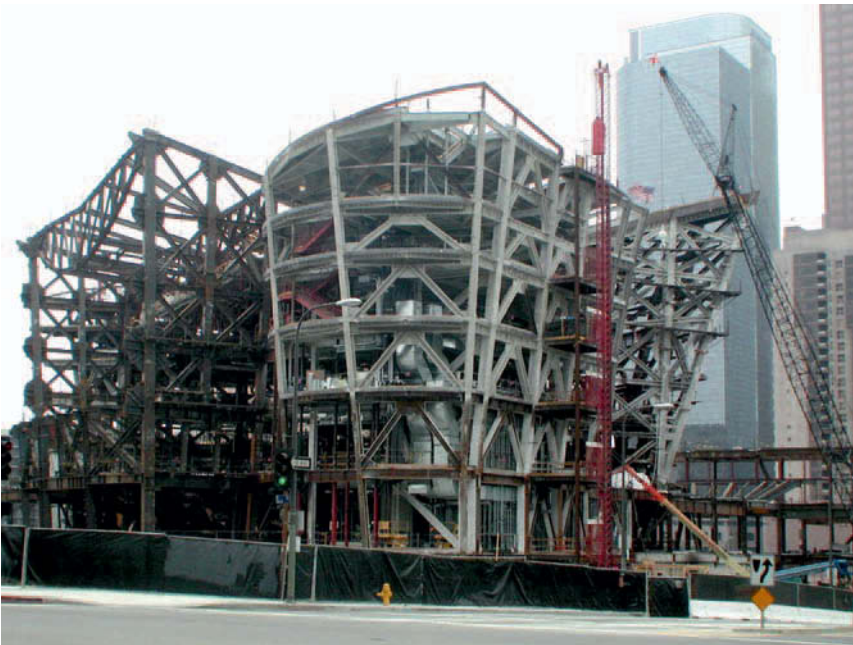
Figure 0.2 Walt Disney Concert Hall, Los Angeles; Frank Gehry (1929–), architect. The supporting structural steel framework is highly inefficient. The overall cost of the building was $274 million, compared to $190 (equivalent) for three other halls on the same site that were built in the 1960s with conventional post-and-beam structures.
